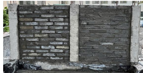
Figure 9. Frame K2 after construction of the infill wall with non-fired solid bricks 40 \times 80 \times 180 mm.
