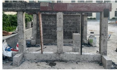
Figure 8. Installation of formwork and reinforcement and casting of the beam at the top of the columns.
