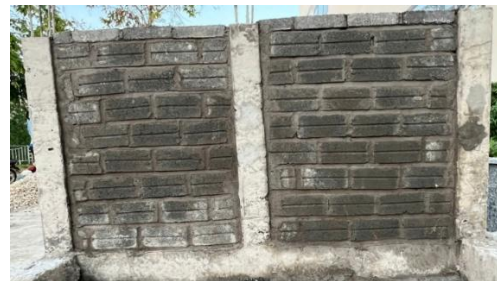
Figure 10. Frame K3 after construction of the infill wall with non-fired hollow bricks 80 \times 80 \times 180 mm.
