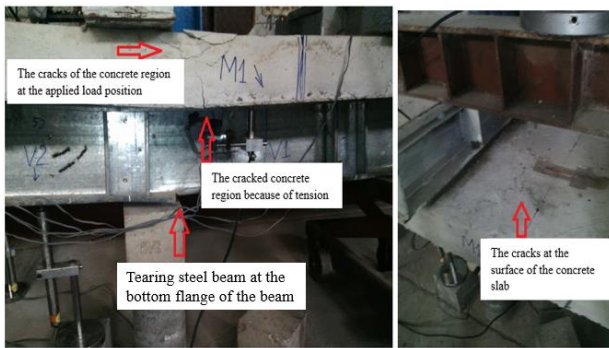
Figure 12. The failure mode of Beam 1.
